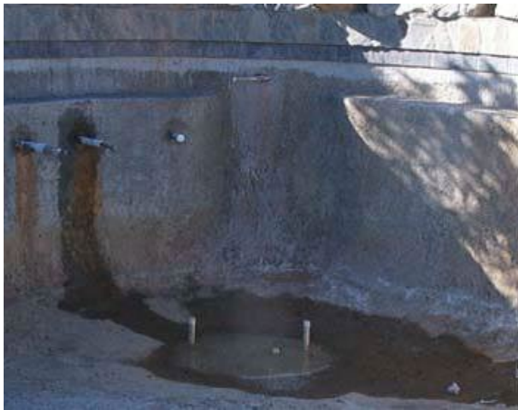
Water from behind the structure prior to application of the interior finish coating.
